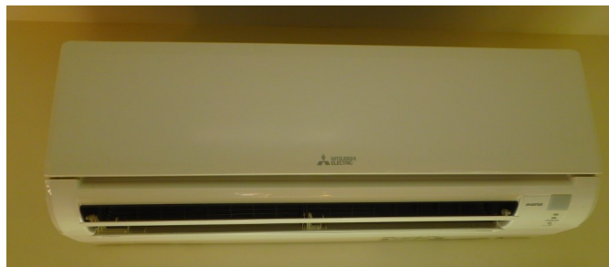
A wall-mounted heat pump head in a residence
